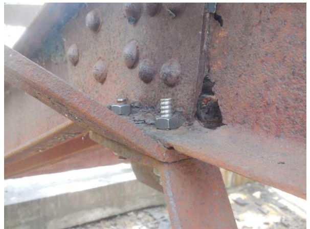
Heads of rusted rivets are removed with a pneumatic rivet buster using a chisel bit and punch bit. Bolts can be easily removed when bridge is dismantled.
