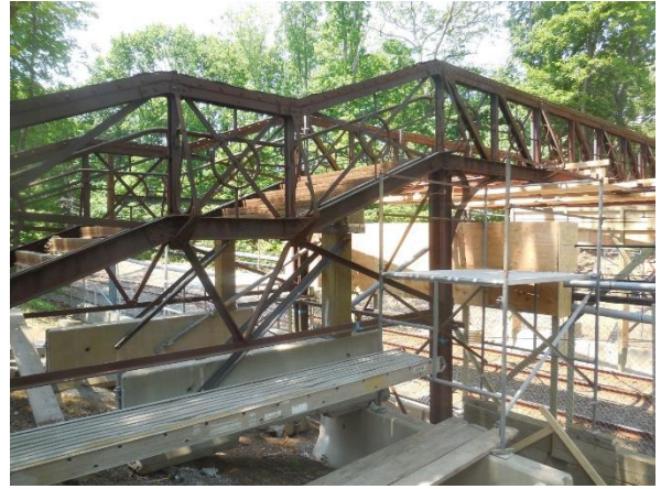
Timbers and concrete Jersey barriers support plywood sheathing to protect against MBTA high voltage power lines
