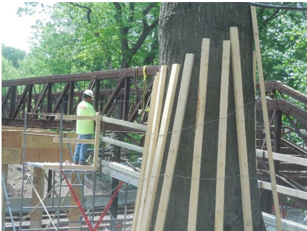
Worker replaces rusted rivets with bolts which can be easily removed when bridge is dismantled.
